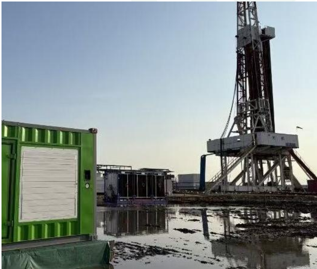
■ 大庆·油田115KWp移动光伏电站 Da Qing Oil Fields 115KWp Mobile Solar Station
